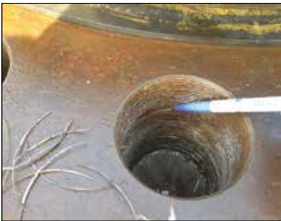
▲ A typical thread before refurbishment
