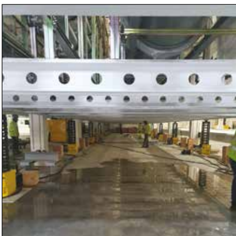
◀ Completed in just over one hour, the 160 ton 50 x 7 meters steel racking system was lifted synchronously to a height of 2,2 meters using 16 Enerpac SCJ50 Cube Jacks powered by a single SFP-Series Split-Flow Pump. Lifting large racking systems can be hazardous, complex and difficult involving forklift trucks and chain blocks. Photo by courtesy of PHL Hydraulics Ireland Ltd.
